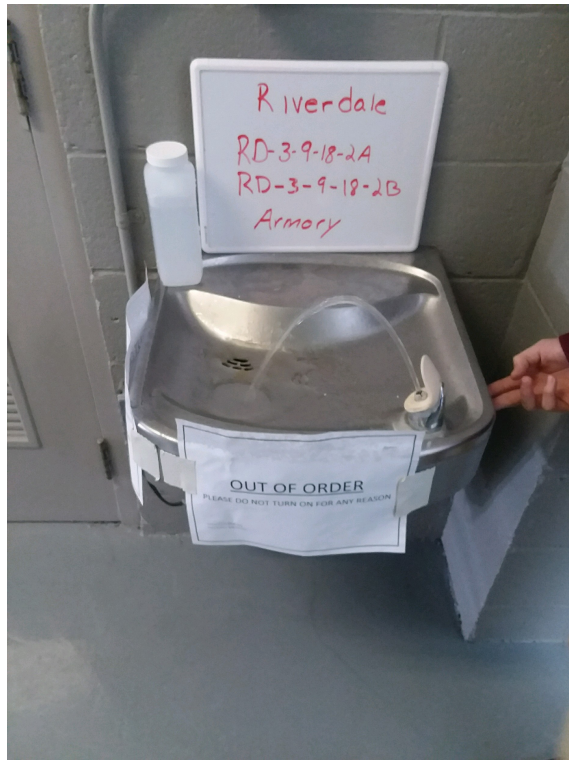
Riverdale Armory 1st Floor Water Fountain
