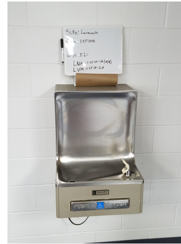
Lawrenceville Marshalls Office Water Fountain
